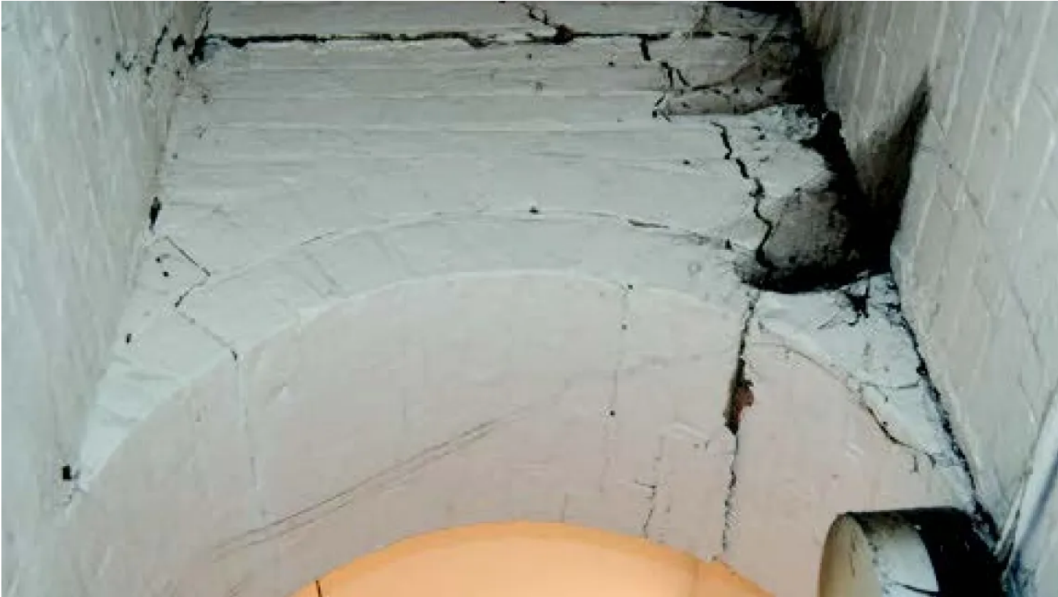
Damage to St Peter-in-the-Forest
